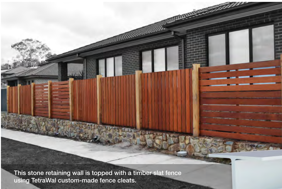
Smooth concrete sleepers are joined with TetraWal H-sections. The Treated Pine piling fence is attached using custom-made fence cleats.
