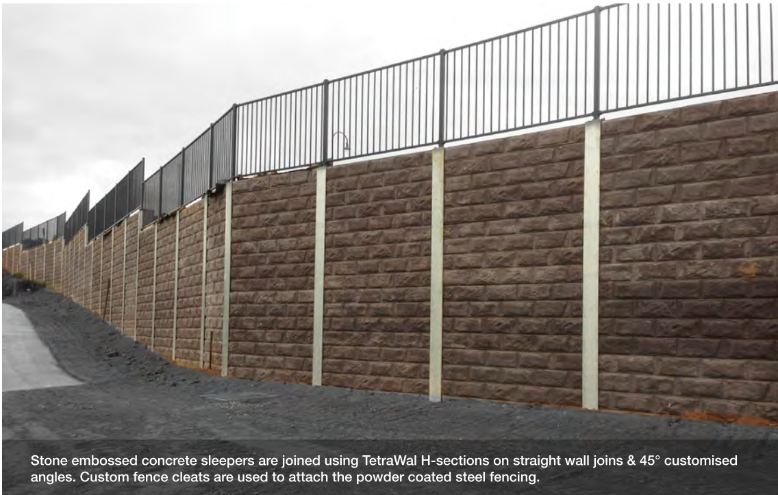
This concrete sleeper retaining wall system uses TetraWal in black Duplex (paint over galvanized steel) H-sections & 45° angles. Custom fence cleats attach the timber railing to the retaining wall.
