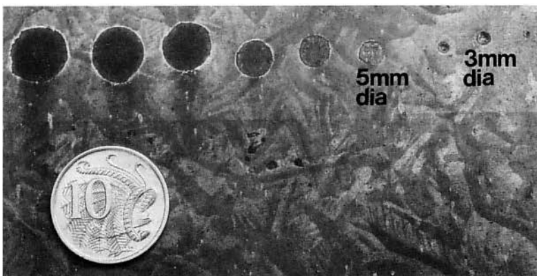
The galvanized steel test piece has had circular areas of the coating removed before exposure in a severe industrial environment. Sacrificial protection is provided by the surrounding galvanized coating and has prevented corrosion of the exposed circles up to 3mm diameter and minimised corrosion of the 5mm circle. Larger circles also exhibit corrosion-free annular areas adjacent to the surrounding coating.
